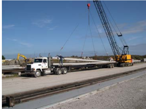
Precast/Prestressed Piles being lifted onto Truck for transportation to another driven Pile project
